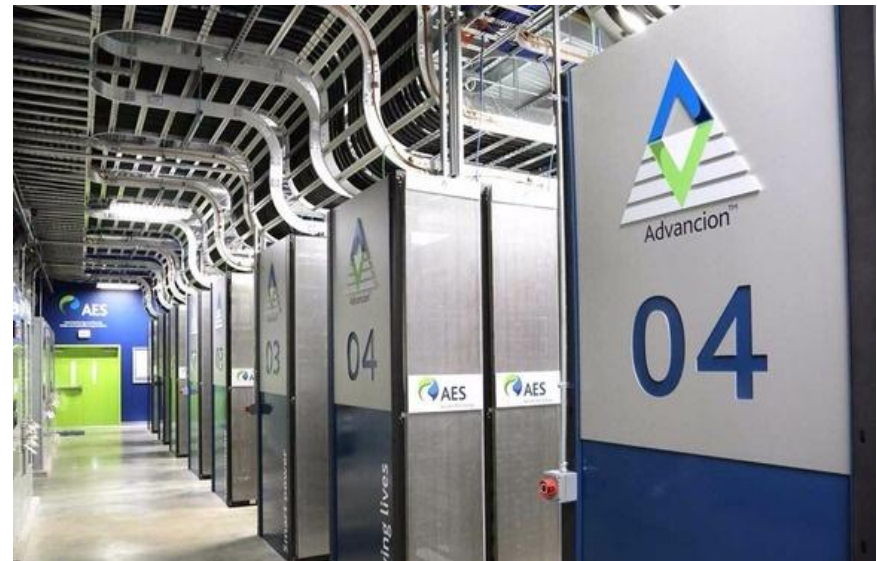
AES Northern Ireland's 10 MW (of 100 MW) BESS
