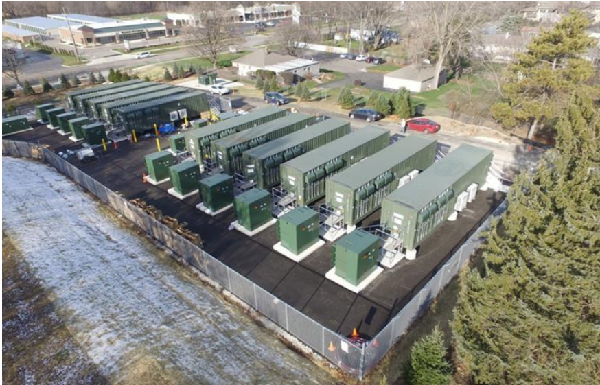
EDF 20 MW BESS (BYD America cells) at Illinois in USA
